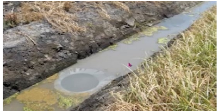
Example of under-seepage in a drainage ditch. DEVERAL, 2023.
